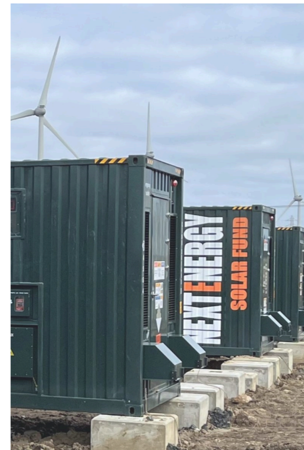
Camilla Battery Storage Asset, NextEnergy Solar Fund
