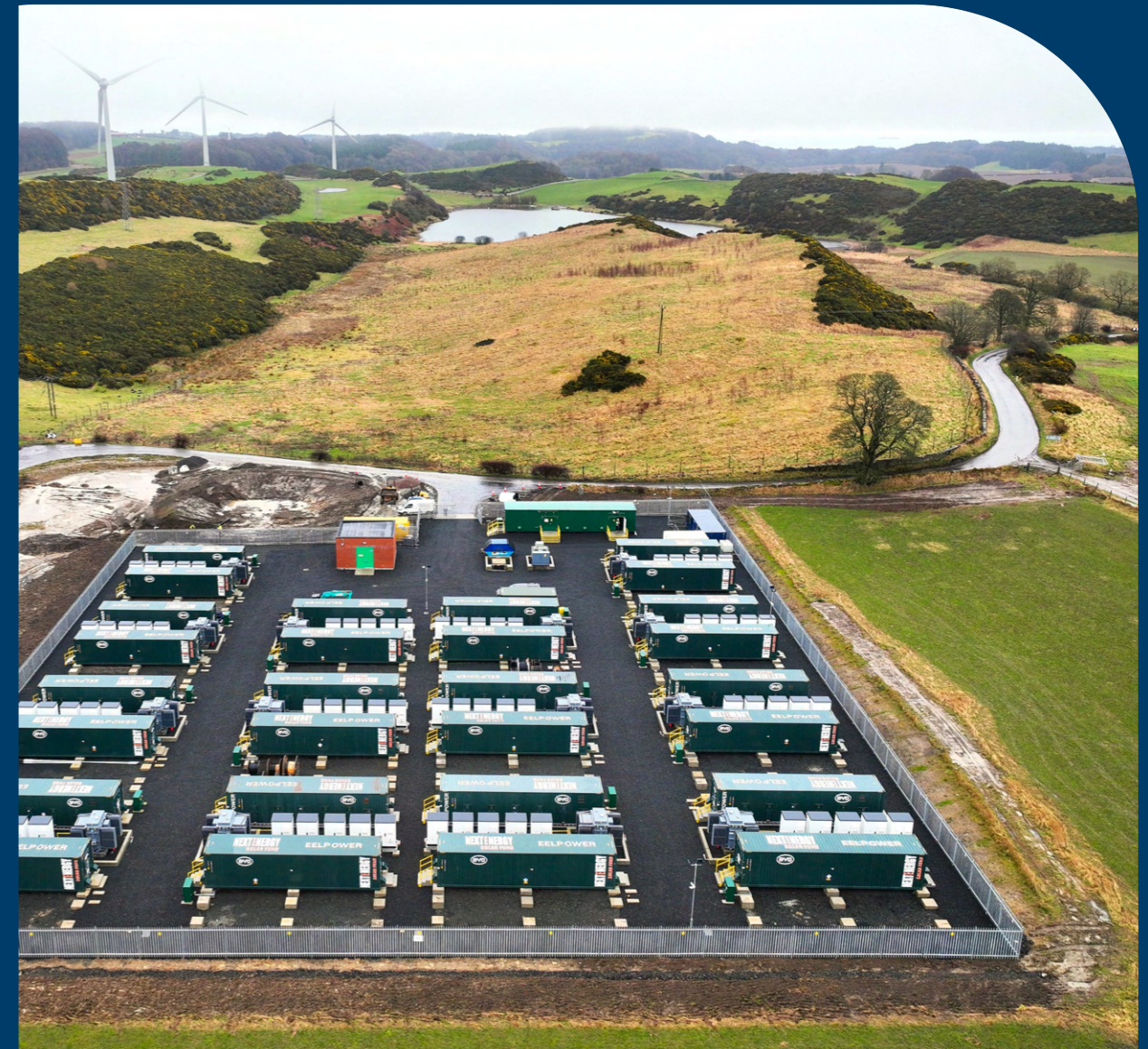
Camilla Battery Storage Asset, NextEnergy Solar Fund
