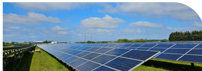
Honington Solar Asset, NextEnergy Solar Fund
